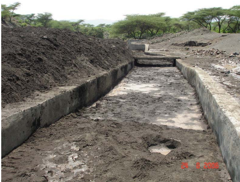
Figure 2. Fokisa spate irrigation scheme main canal (capacity reduced as a result of sedimentation)
